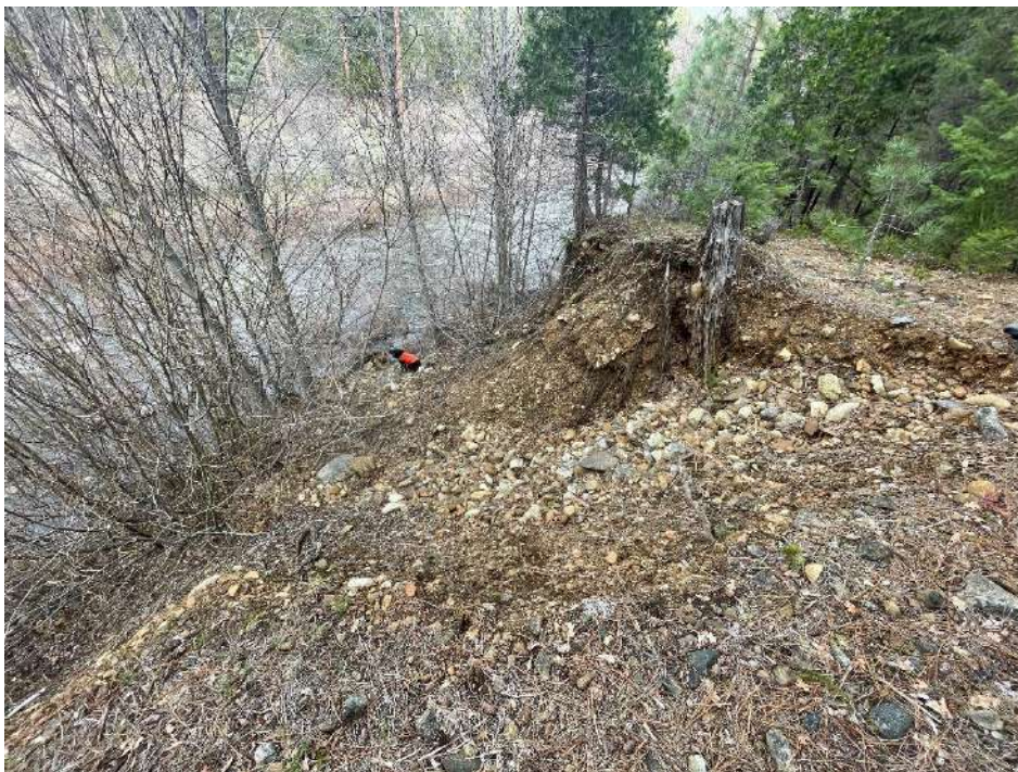
Photo 2.32: Deep incision where EFG 8.3 discharges into the East Fork Scott River. EFG9. April 5, 2024.
