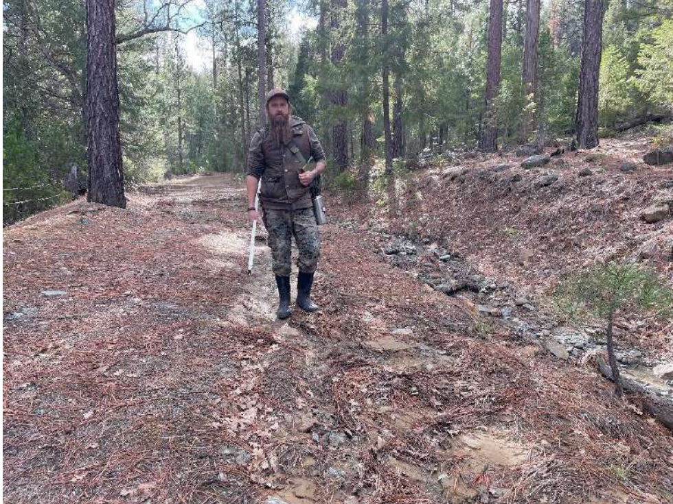
Photo 2.10: Flow divided between road and un-engineered inboard ditch. EFG2e. January 19, 2024.
