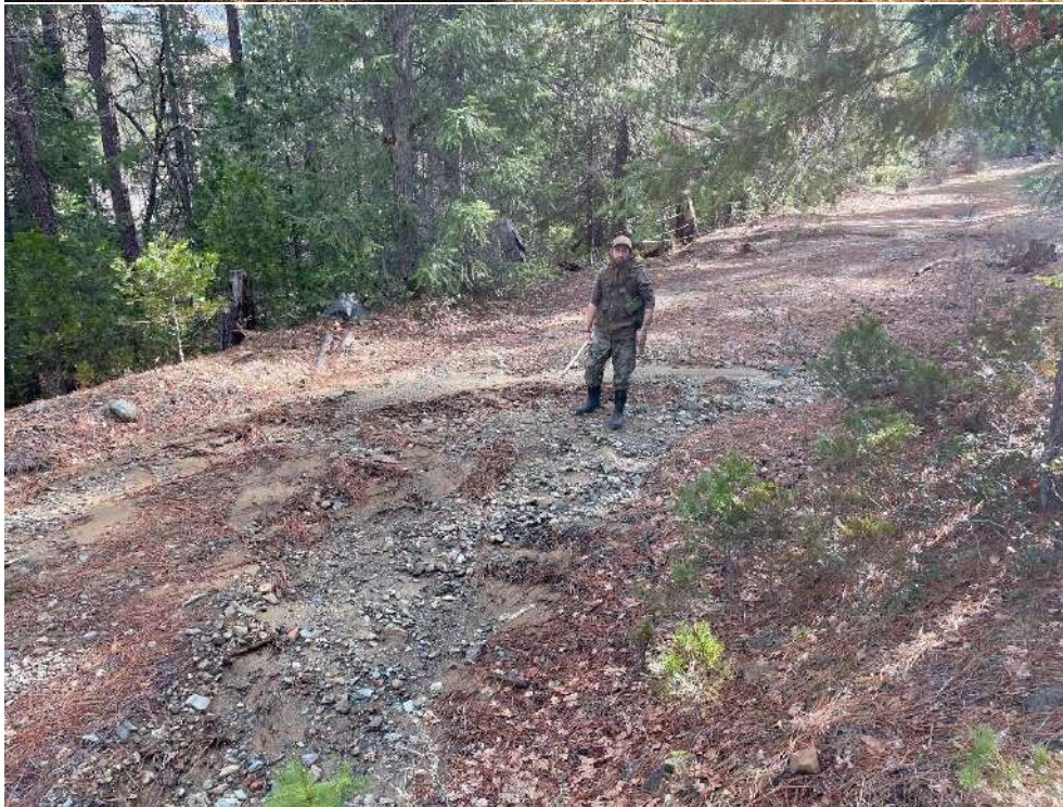
Photos 2.8 & 2.9: Flow path on road. EFR14; January 20, 2023. EFG2e. January 19, 2024.
