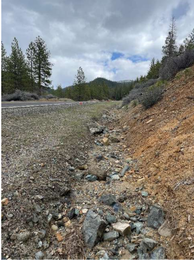
Photo 2.50: This inboard ditch on Highway 3 is the source for EFG 24. EFG24a. April 5, 2024.
