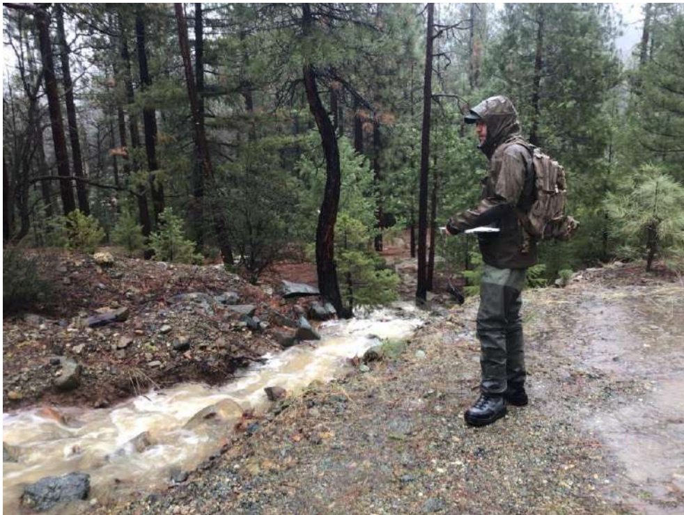
Photo 2.6: Erosion of road fill. EFR2. January 13, 2023.
