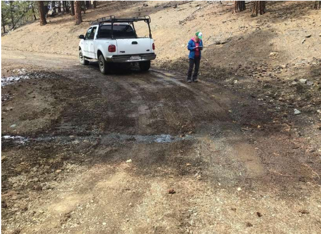
Photo 2.1: Example of mild erosion point. HRR20, April 18, 2023.
