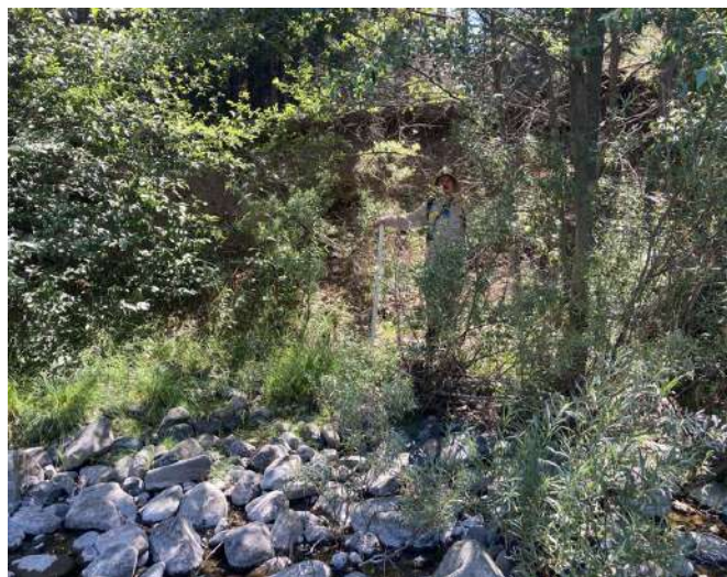
Photo 1.4: Severe erosion site located at transect EF-14. September 1, 2022.
