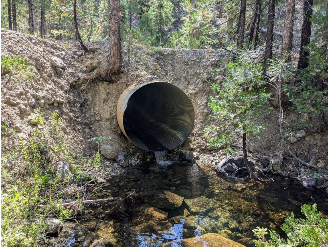
Figure 4-53. The outlet of STX-7. Severe erosion of the road fill prism is evident.
