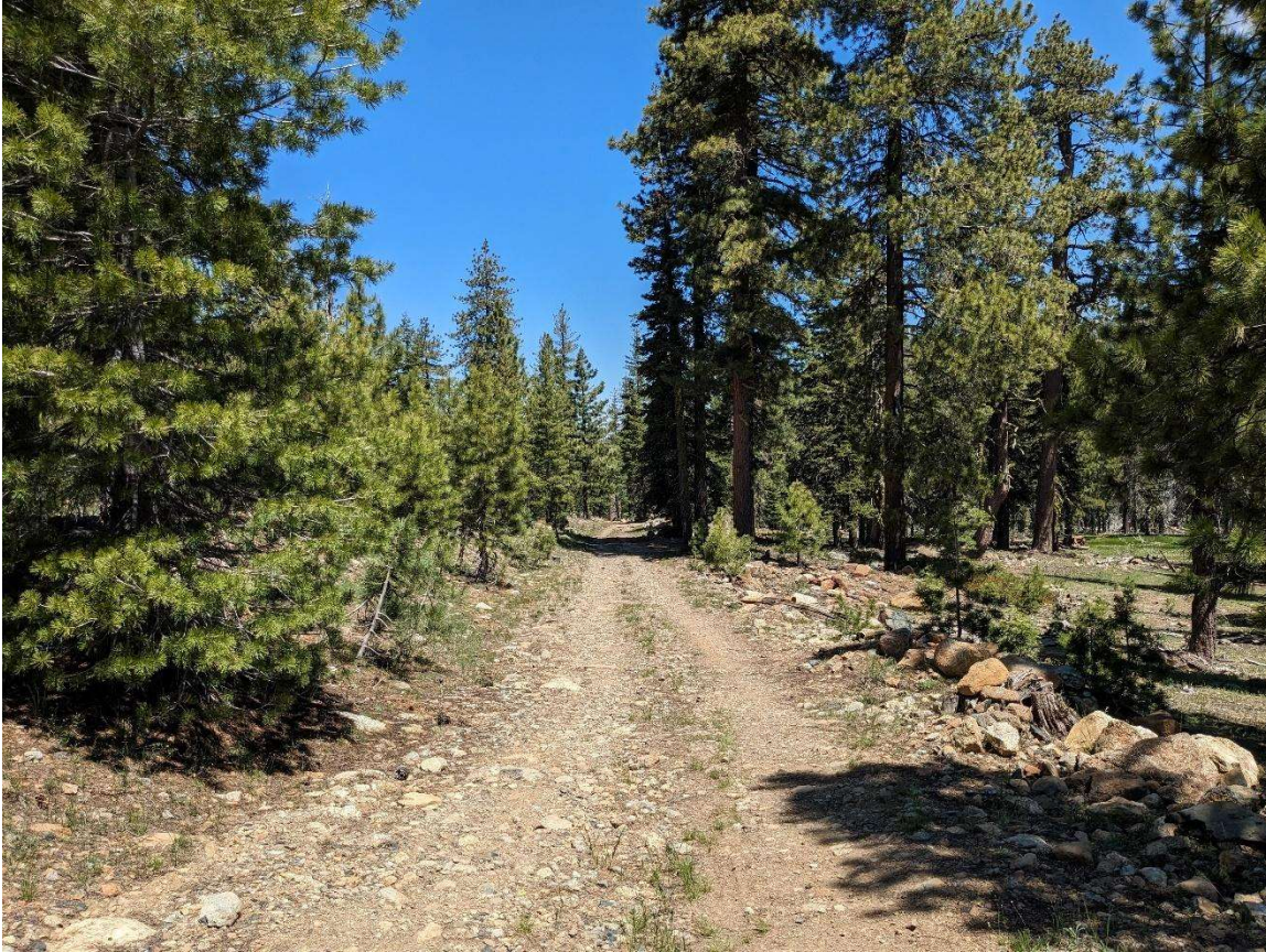
Figure 4-51. A representative section of road segment RF-2 looking north, showing the generally flat road profile and outboard berm which tends to concentrate flow from the western hillslope.
