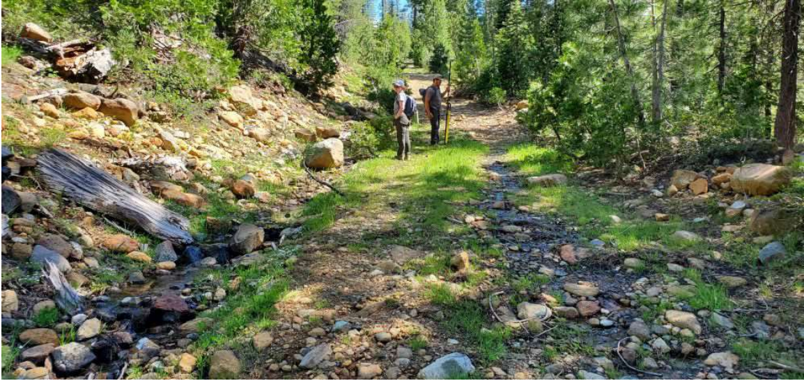
Figure 4-45. Looking upslope at road segment CM-8, with active flow visible in the inboard ditch to the left, as well as on the road surface to the right.
