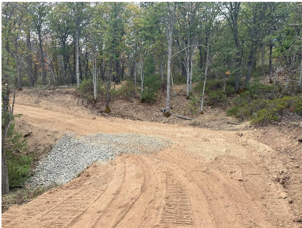
Drainage crossing on west dozerline – see pg 30
